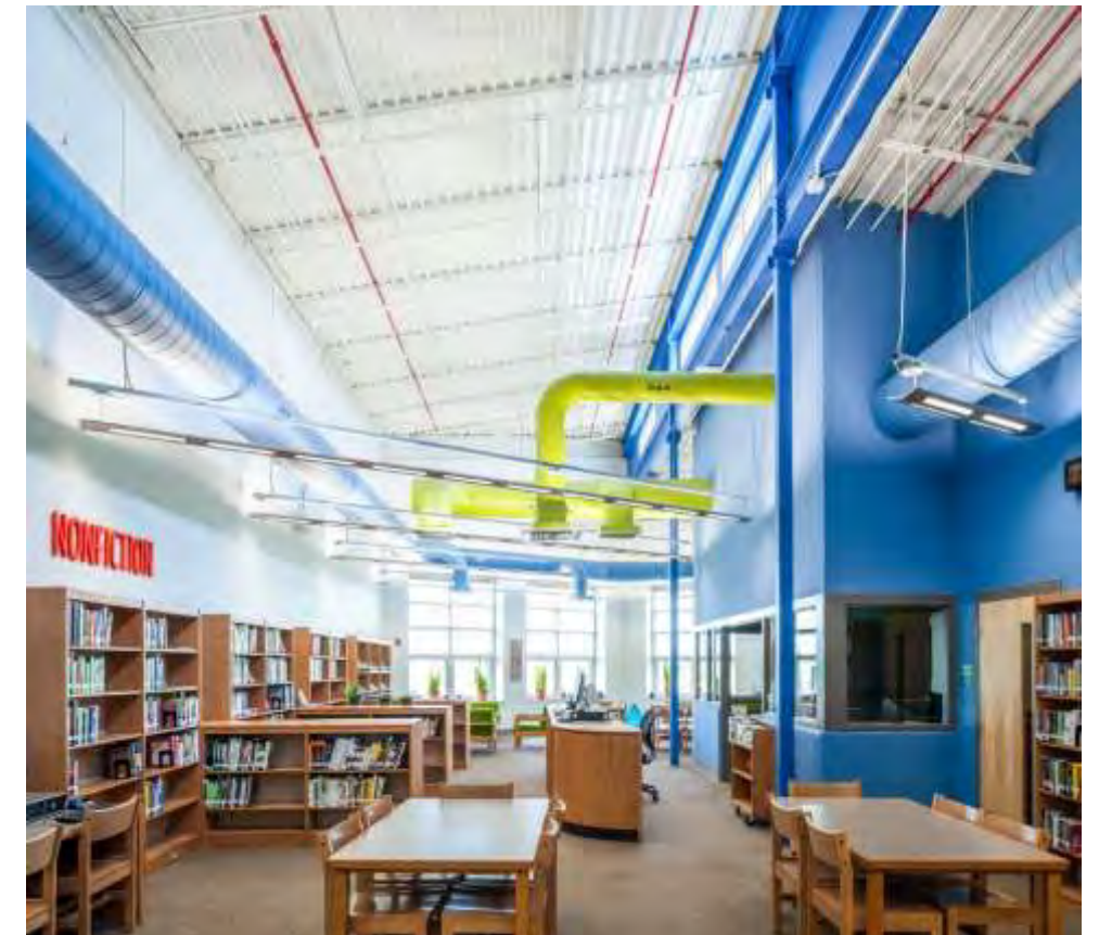
Image Credits: CMTA Engineers
