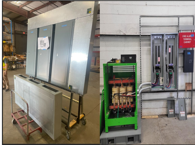
Prefab Electrical Closet
